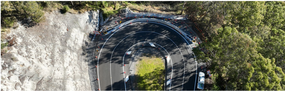
DRFA 22A Urgent REPA – Lamington National Park Road, QLD, Australia.
