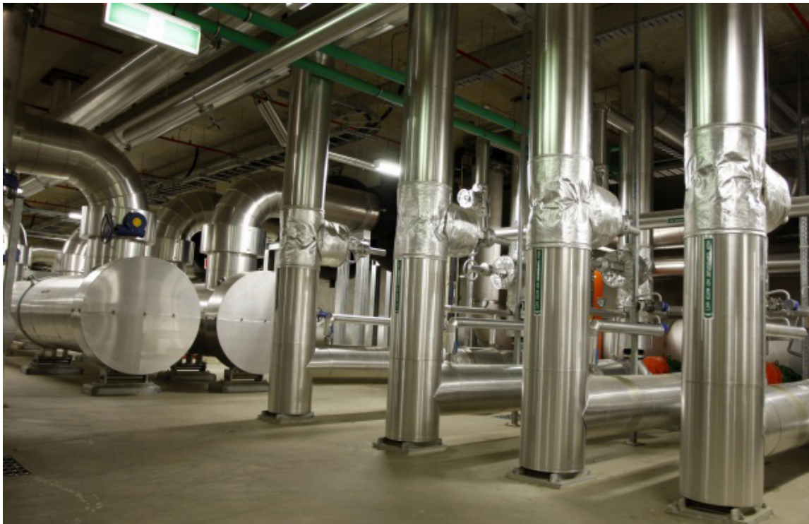
Queen Elisabeth II Central Energy Plant – Nedlands, WA, Australia.
