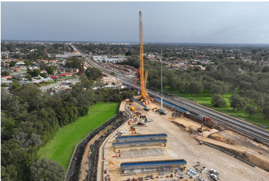
METRONET Thornlie-Cockburn Link & Yanchep Rail Extension, Canning River Rail Bridge - Perth, WA, Australia.
