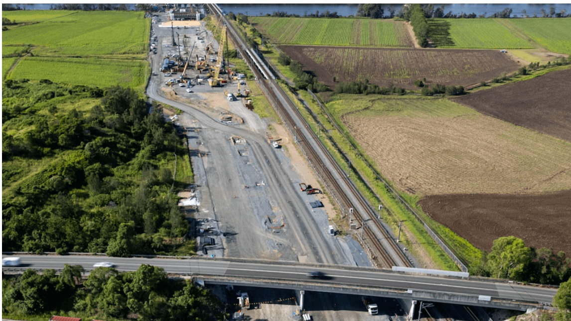
Coomera Connector (Stage One North – Shipper Drive to Helensvale Road) – Gold Coast, QLD, Australia.
