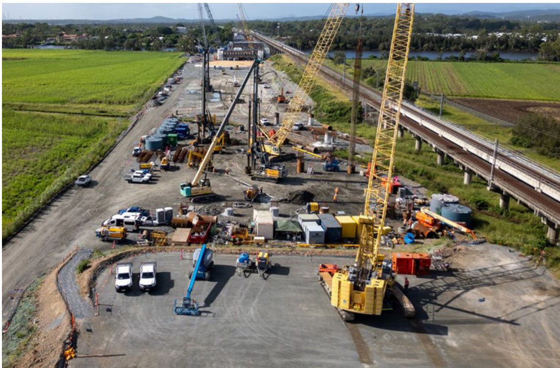
Coomera Connector (Stage One North – Shipper Drive to Helensvale Road) – Gold Coast, QLD, Australia.
