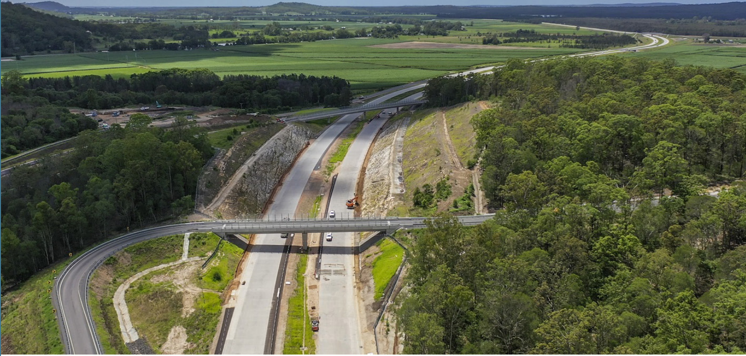
Pacific Highway Upgrade, Woolgoolga to Ballina - Portion A - North Coast, NSW, Australia.
