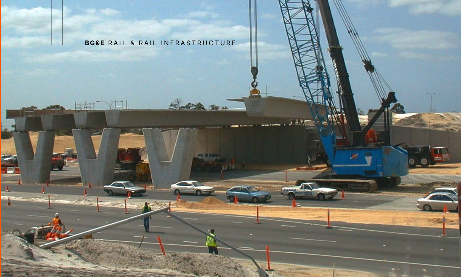
Kwinana Freeway Interchanges & Extension — Berrigan Drive-to-Safety Bay Road — Freemantle & Rockingham, WA, Australia.
