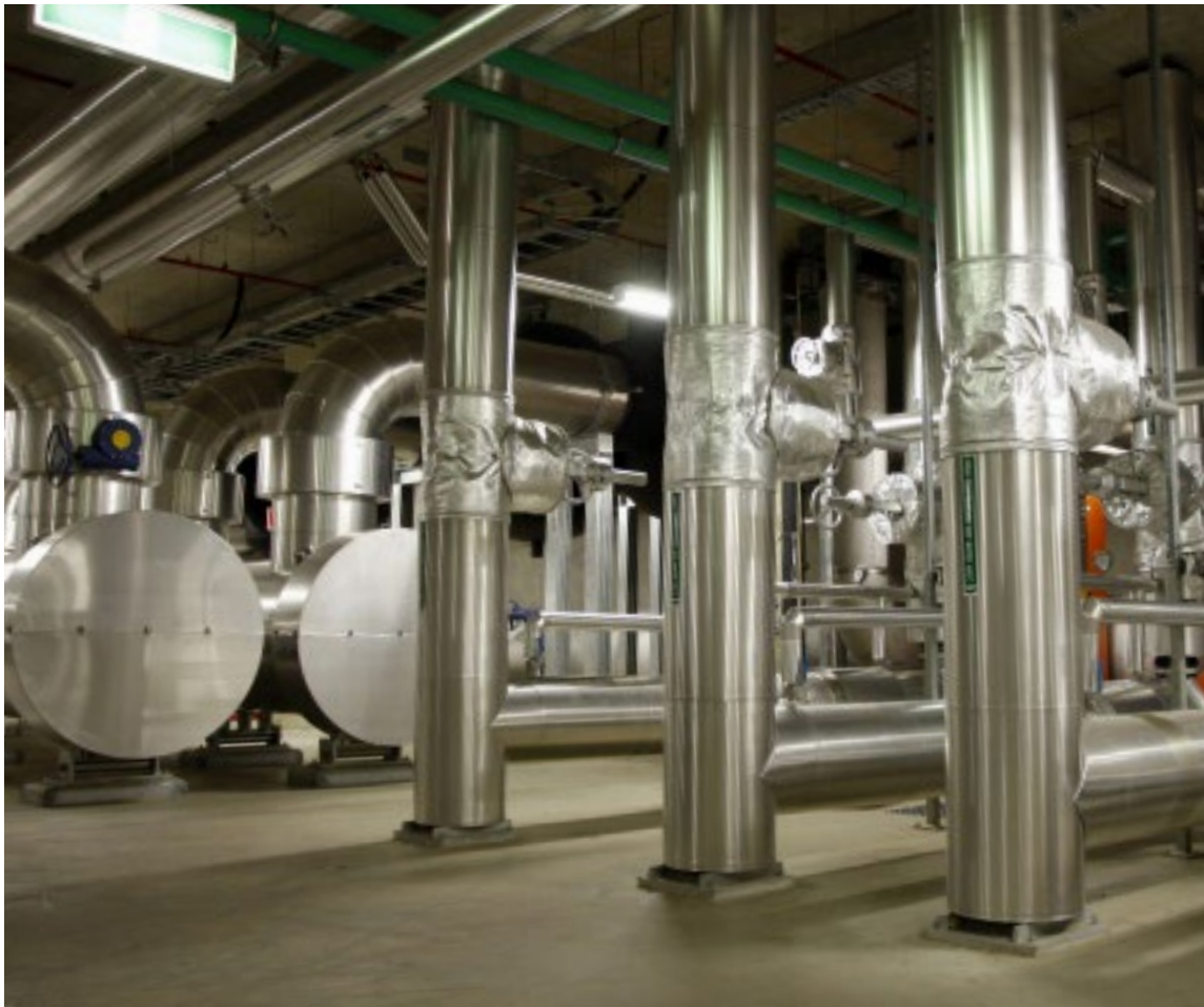
Queen Elizabeth II Central Energy Plant — Nedlands, WA, Australia.
