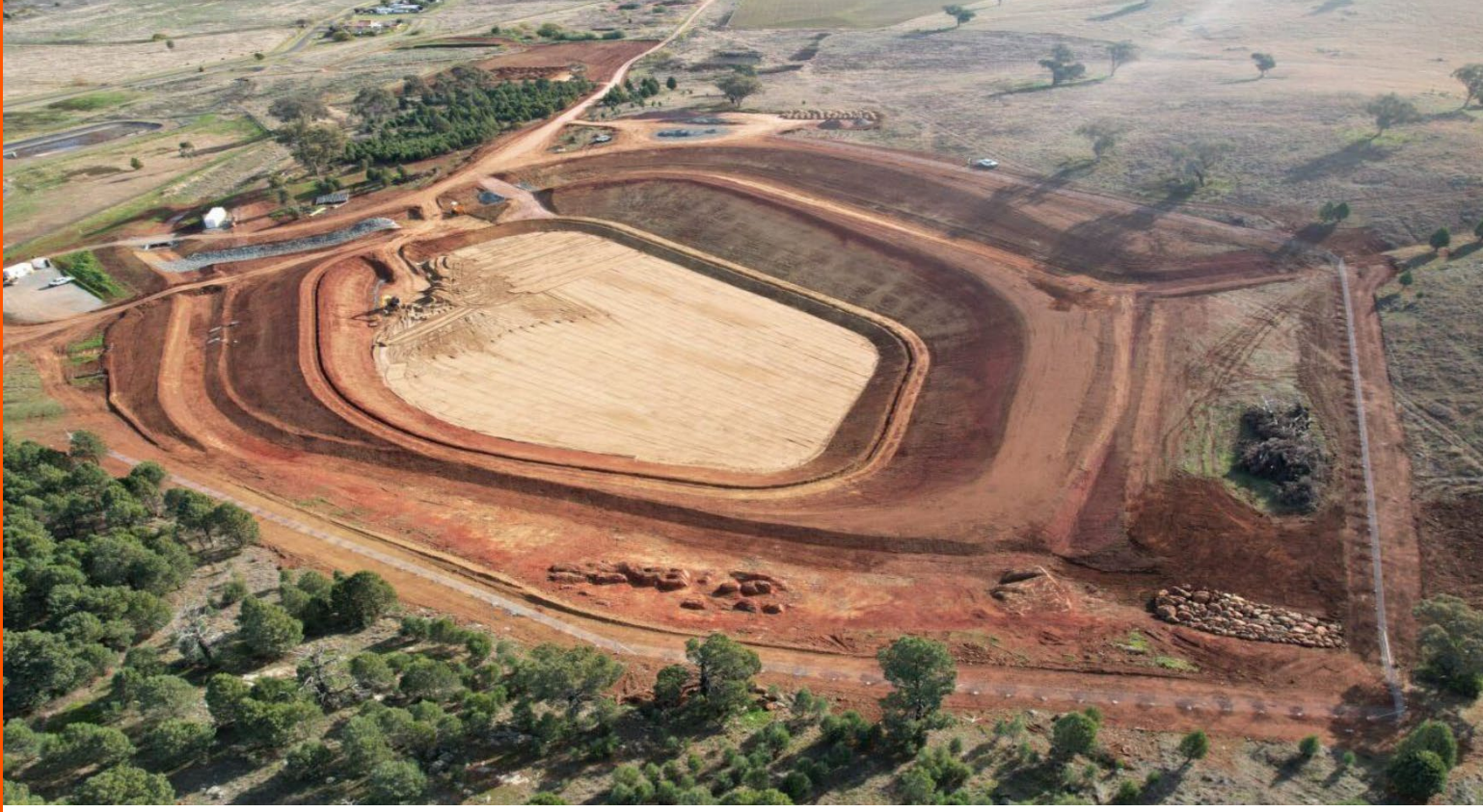
Parkes Flood Mitigation & Surface Water Assessment — Parkes, NSW, Australia.
